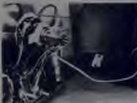
Inside of monitor, showing outlet socket installation.
